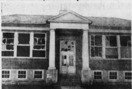
Lehigh consolidated school in which 13 children and two teachers were injured by the blast at Sandts Eddy quarry. The school was ordered closed until a thorough investigation is made to determine how badly the building is damaged.
